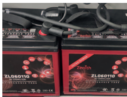
AGM batteries compartment
